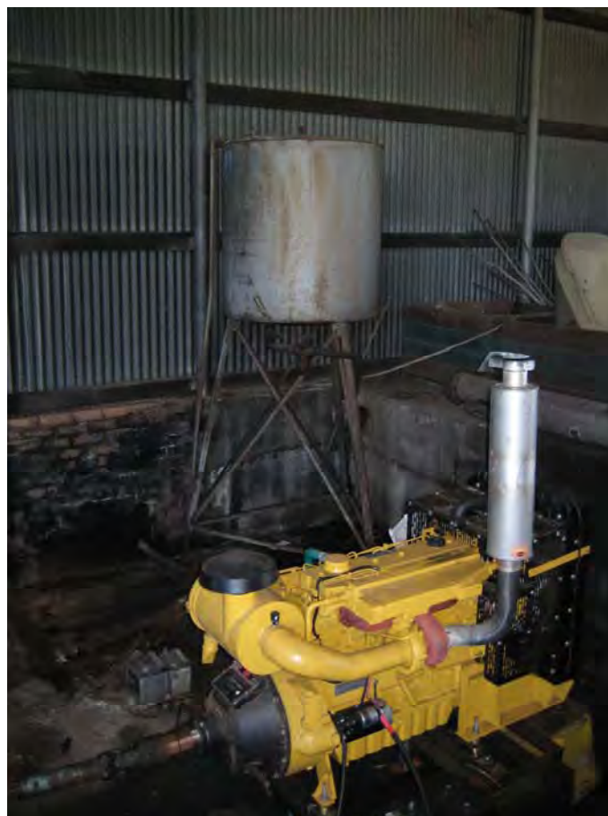
PLATE 10 – Petrol tank and motor for well in shed on Lot 14 Kerosene Lane, Baldivis.
