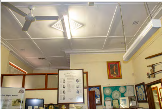
ceiling vent and cover batten
